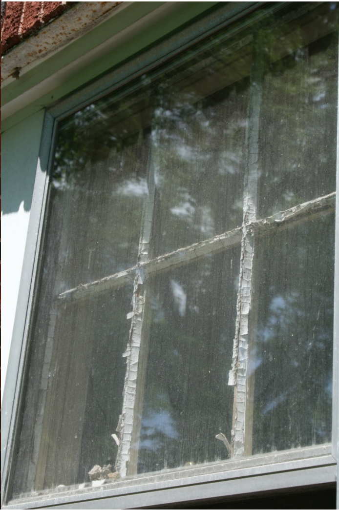
Glazing Falling Off
